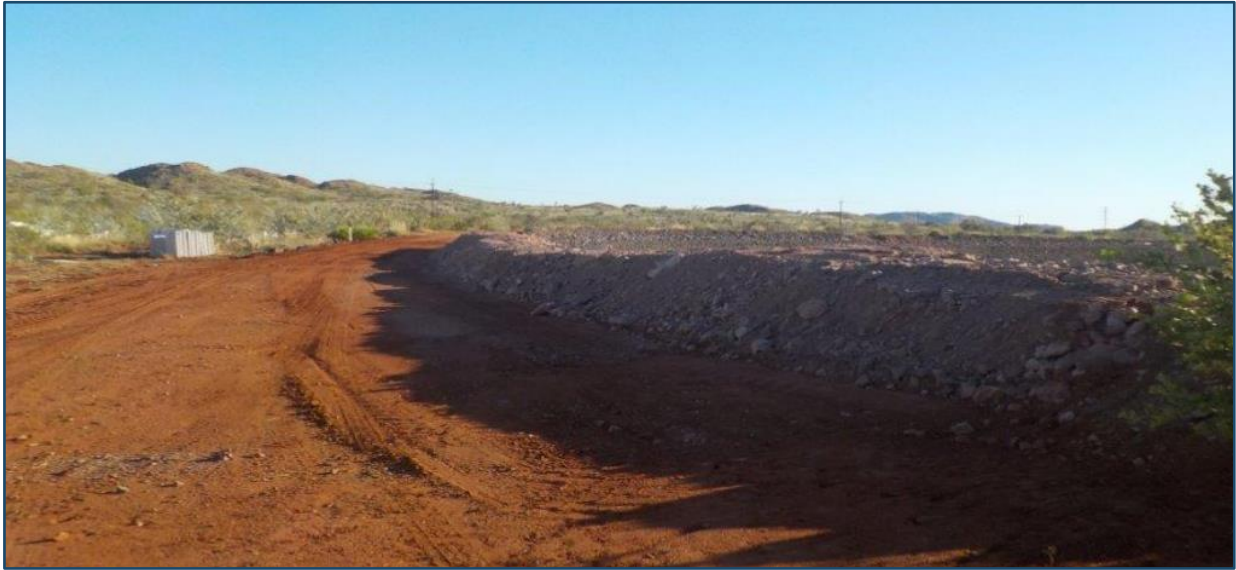
Figure 4: An example of recently constructed bunding aimed at diverting storm water run-off away from existing infrastructure
